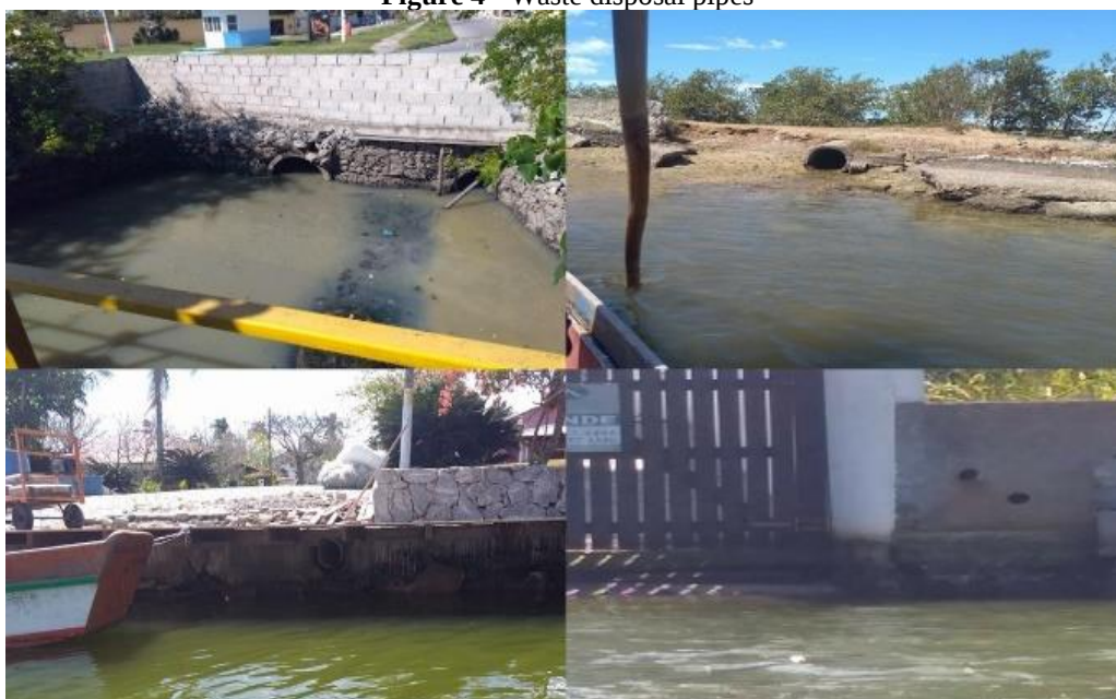
Figure 4 - Waste disposal pipes
